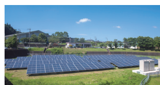
150 kW photovoltaic power generation system (Grid 2) Site: Rear of Yusuin health center
